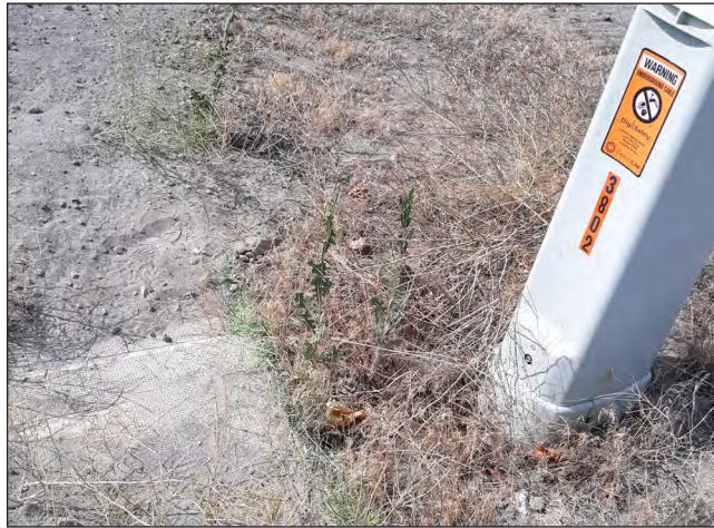
PHOTO 5: Underground cable warning post
